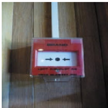
Fire alarm button
