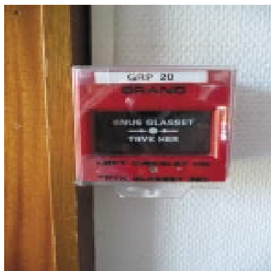
Fire alarm button
